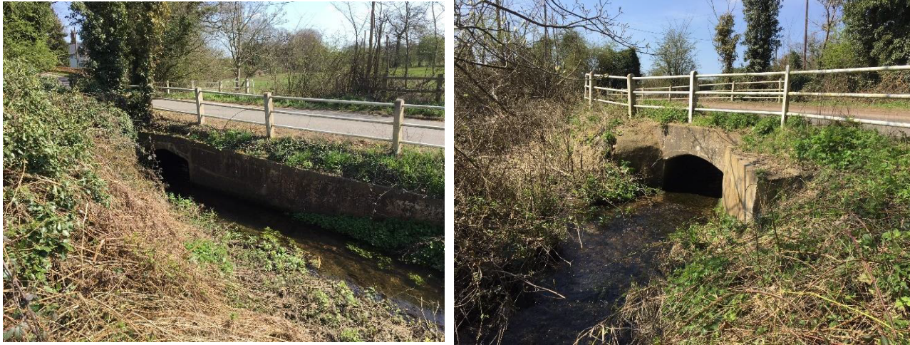
Figure 2-2: Photographs upstream (left) and downstream (right) of existing Cantley Lane South culvert
